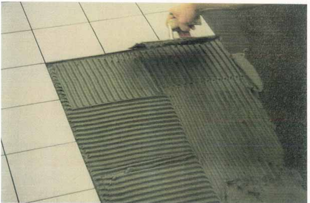
Picture 3 – The mortar and the clinkers during assembly. The clinkers were 7-8 mm thick.
