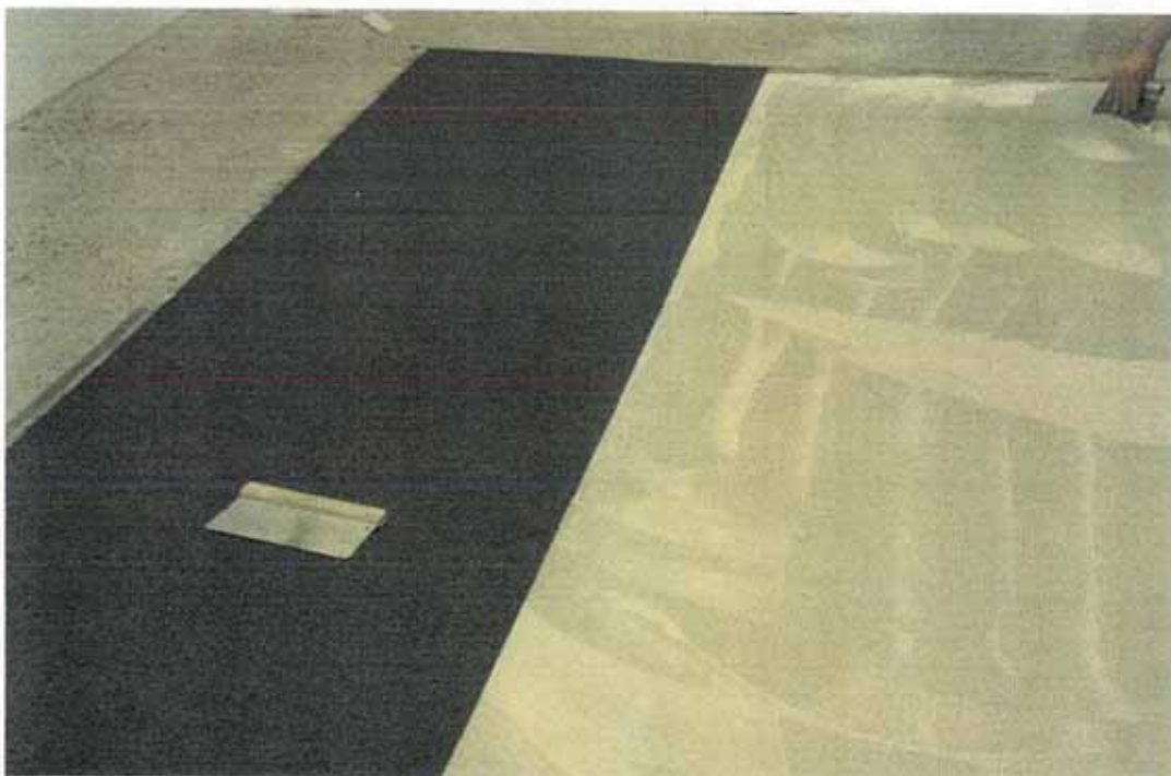
Picture 1 – The underlay of the flooring were glued on the laboratory concrete floor slab.
